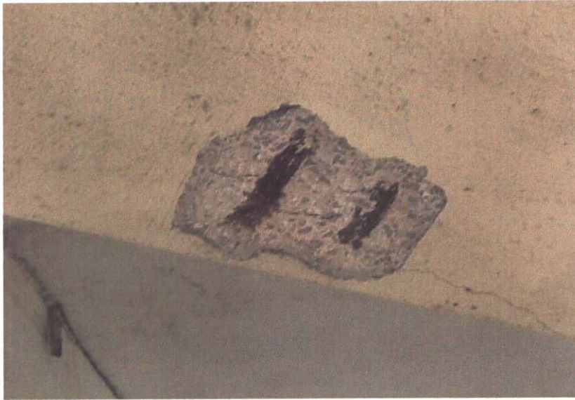
PIER #2 POP-OUT WITH EXPOSED REBAR ON BOTTOM
