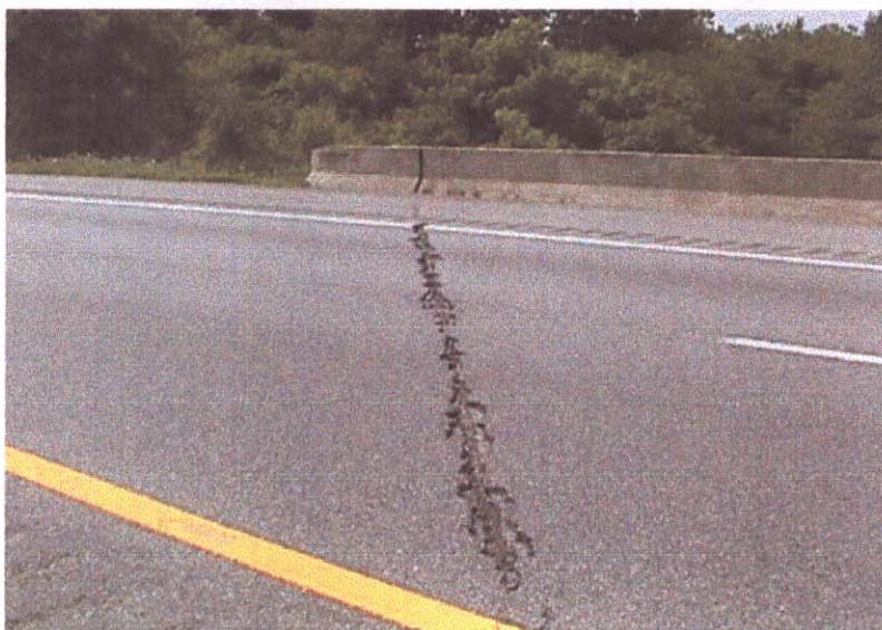
POTHOLES @ JOINT B-APPR-TYPICAL
